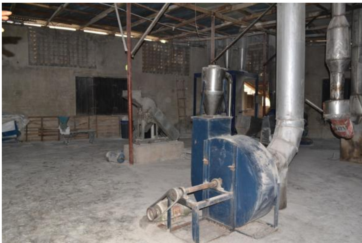
Figure 4: Matsol flash drying plant, Ogun State
