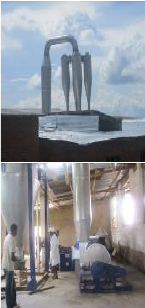
Figure 37: Drying of HQCF using a flash dryer (2-10t/shift)
